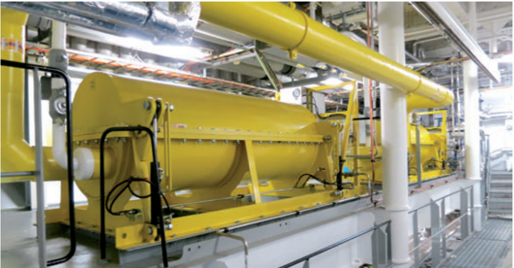
Wärtsilä Gas Valve Unit Enclosed Design (GVU-ED™) installed directly in the Engine Room
