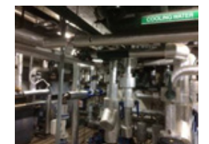
typical building plant room
